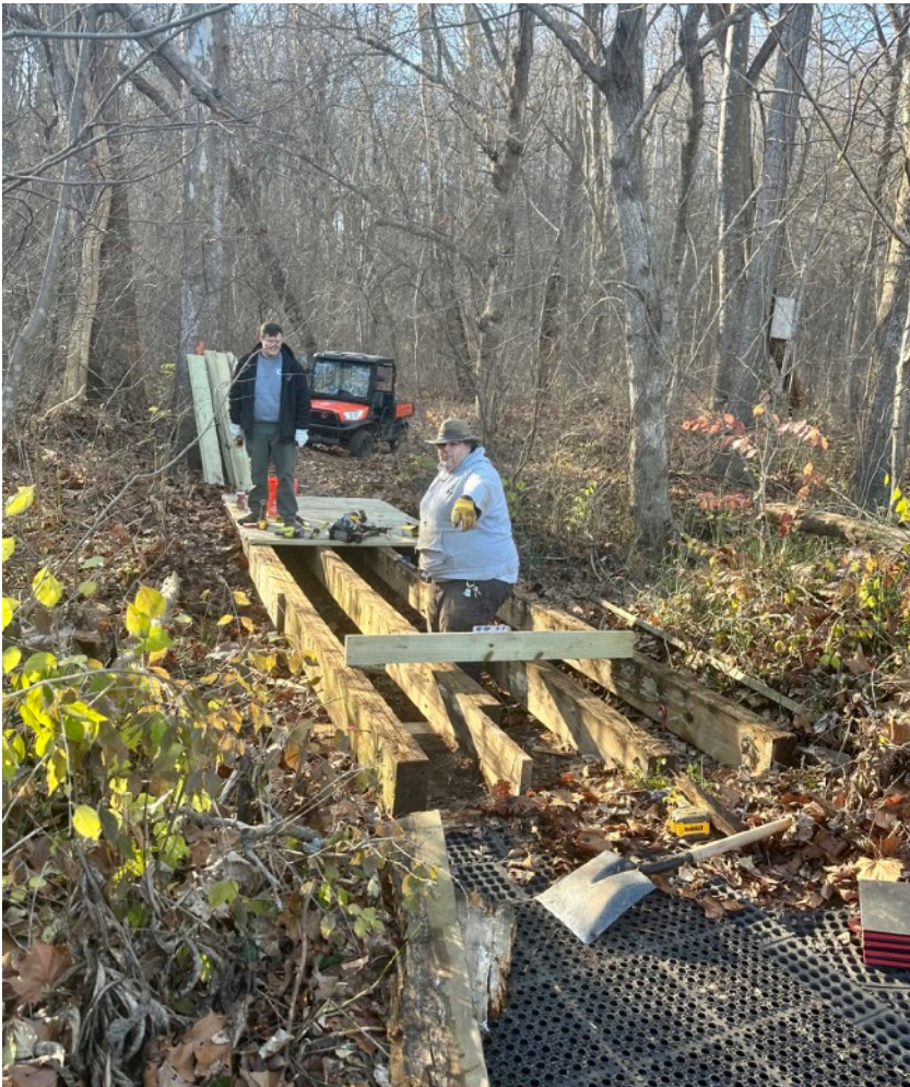
Casey Pittrizzi, Natural Resource Manager, and Matt McNeal, Maintenance Crew Chief, working on the bridge on the Follow the Hollows Trail
